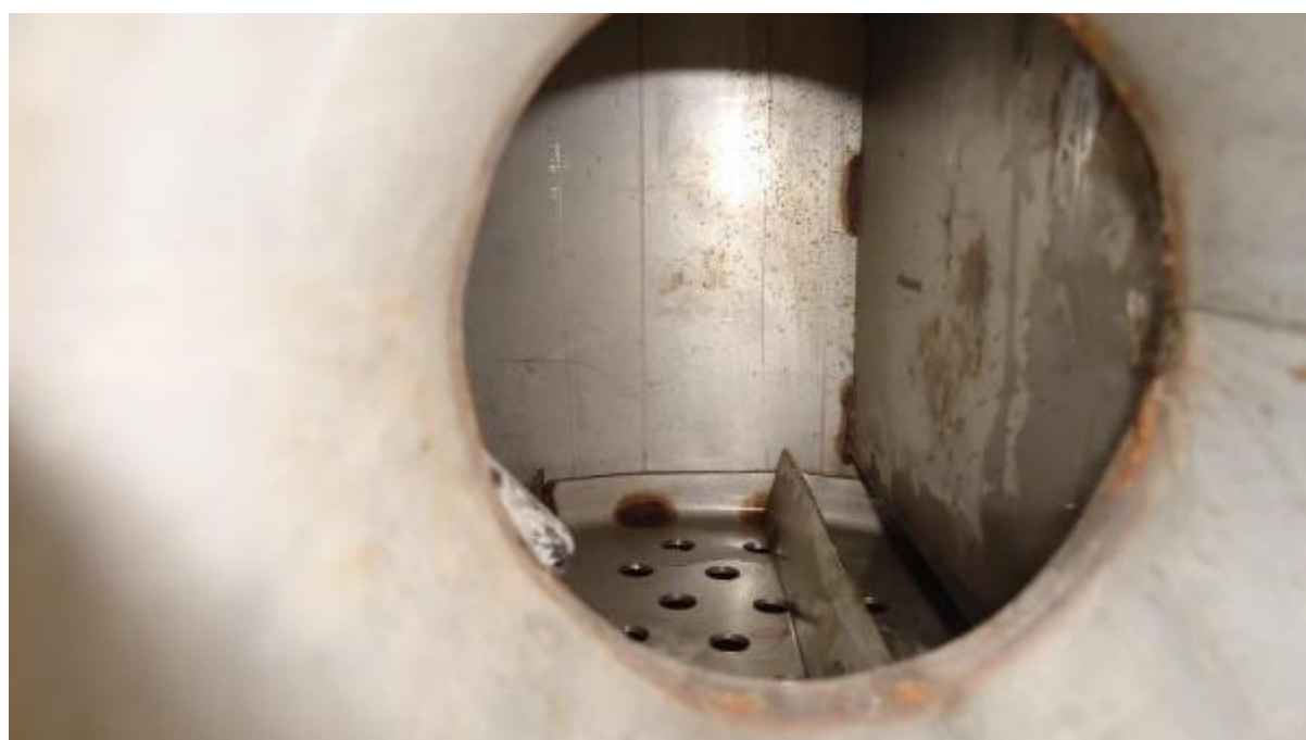
Inside the distillation column/tray
